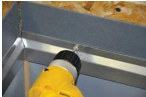
Image 27: Pre-drill using 1/8” drill bit. Use screws and anchors appropriate for wall type.
